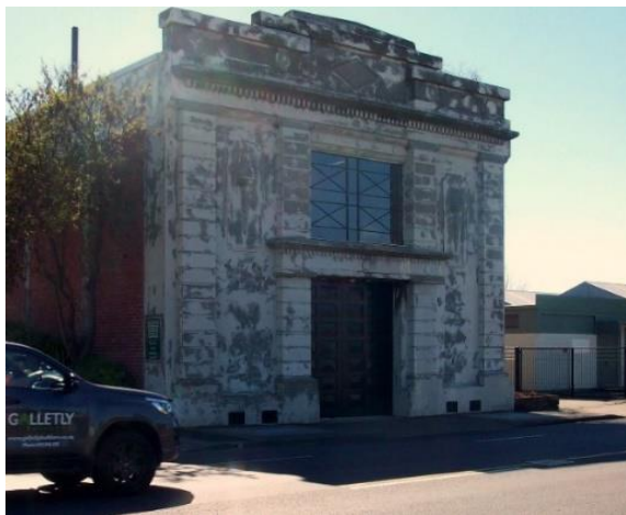
Milton St Substation
